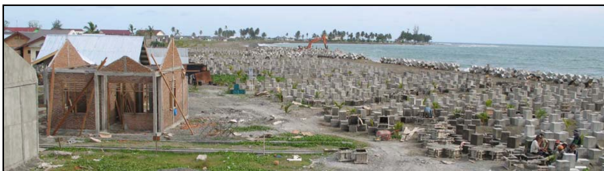
BUILDING OF EROSION CONTROL WALL ON THE MEULABOH PENINSULAR – THIS BREAKER WILL NOT PROTECT THE HOUSES AGAINST A TSUNAMI.
