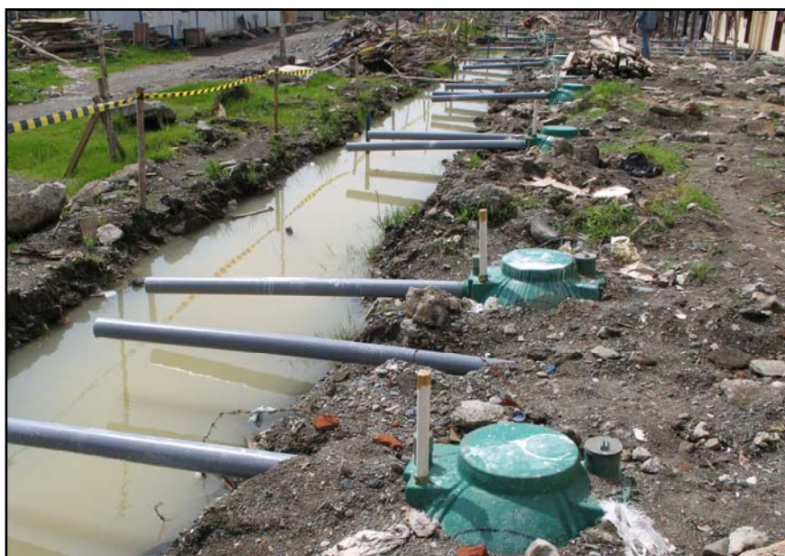
SEMI-DIGESTED EFFLUENT FROM MANY SEPTIC TANKS WILL BE DISCHARGED INTO THE OPEN DITCH WHEN THE HOUSING (RIGHT) IS OCCUPIED. CURRENTLY THE DITCH DOES NOT DRAIN PROPERLY DUE TO THE EARTHQUAKE. WHEN THESE ISSUES ARE NOT RESOLVED, DISEASES WILL BE THE RESULT.
