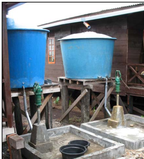
GOOD APPLICATION OF RAINWATER HARVESTING, COMPLEMENTED WITH A SHALLOW WELL FOR WASHING WATER
