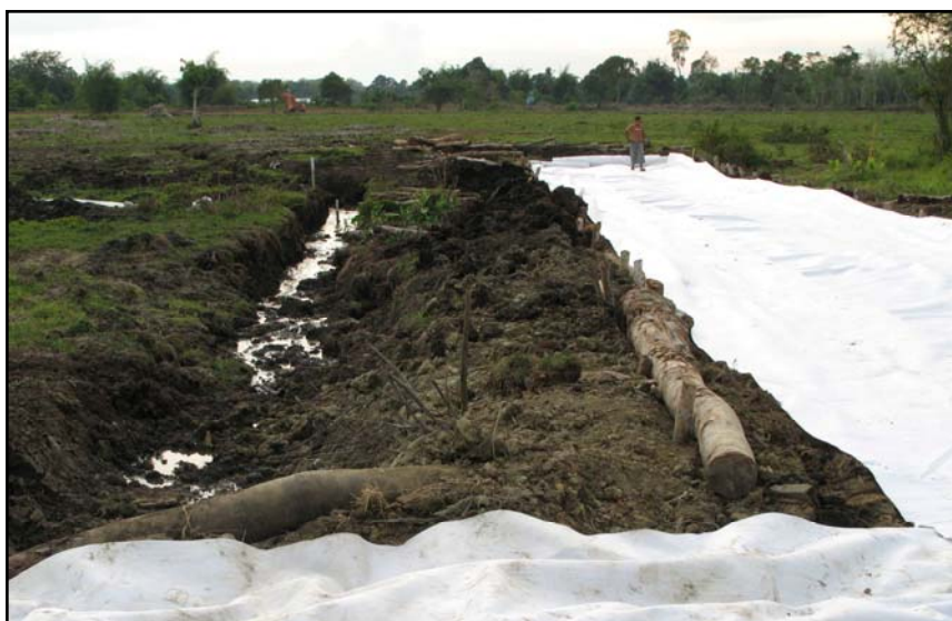
LAYING OF A ROAD FOUNDATION CLOTH ON SWAMPY SOIL BY THE NGO
